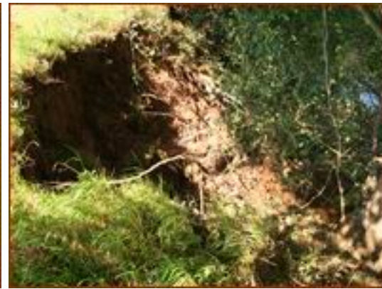
Big scour hole in need of repair, and willow in need of coppicing!
