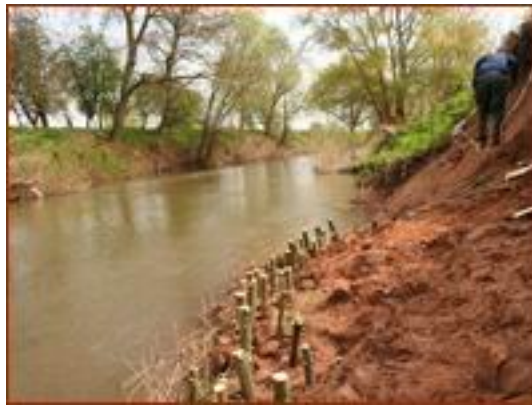
Willow stakes may help with erosion of this scourhole
