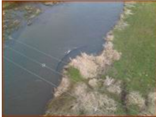
Aerial view of croy needing repair; somewhat eroded behind!
